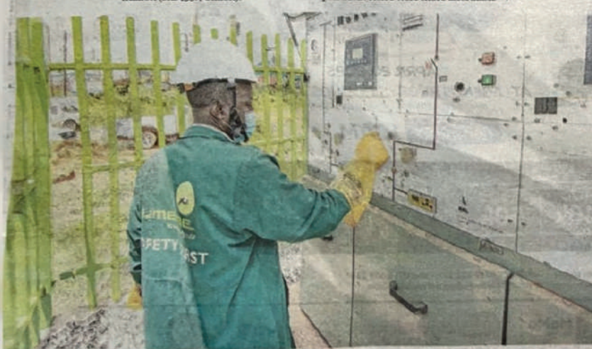
worker at Umeme's Ring Main Units in Namanve last year. PHOTO/FILE
